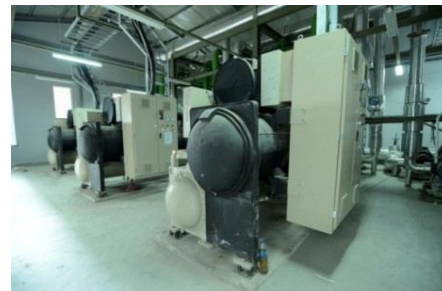
Gambar. 2. Chiller Water Cooled Centrifugal Daikin
