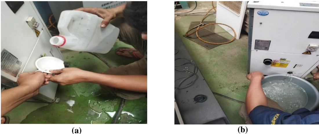
Gambar 6. Dokumentasi Preventive Maintenance Water Chiller
